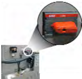
Fig. 12: Power switch (in "OFF" position)
