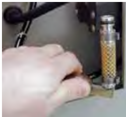
Fig. 56: Water filter loosened
